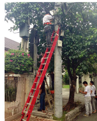
Outdoor Pole Termination
